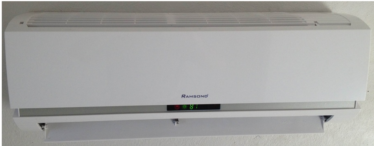
Figure 2.2.4: Ramsond SEER-13 one-ton ductless heating and cooling heat pump; AC power 120 volt current meters installed on main power line driving both fan and heat pump functions.
